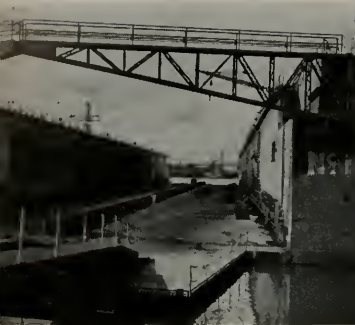
Setting foundation blocks on bottom of drydock. Ship will eventually be supported by these blocks. They have to be aligned in such a manner as to conform to the vessel's underwater body shape. Drydock engineer is setting heights of blocks with surveyor's transit.
